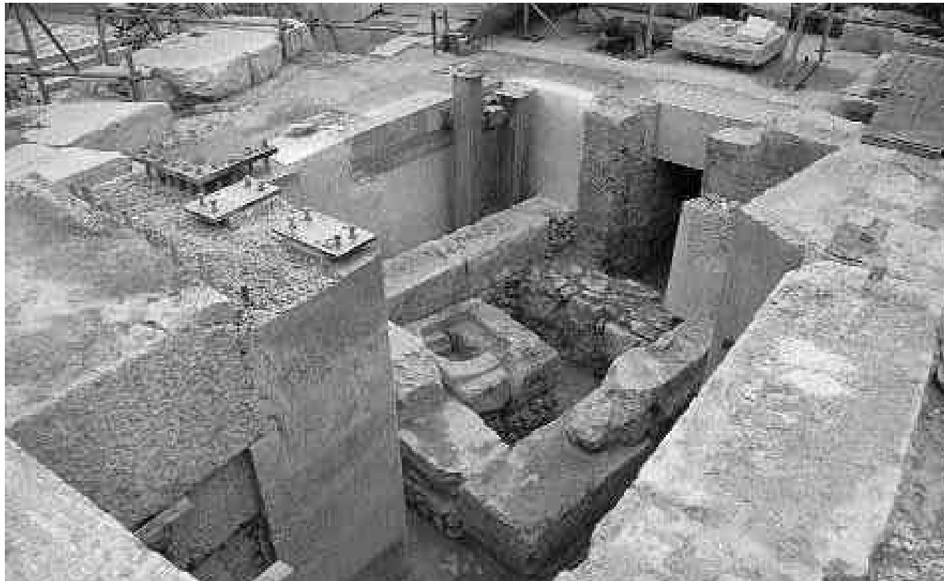
Preparation for placing the stainless steel grid in the bastion of Athena Nike. Inside the bastion are visible the relics of the classical poros naiskos. Photo K. Maloungas, 2004
