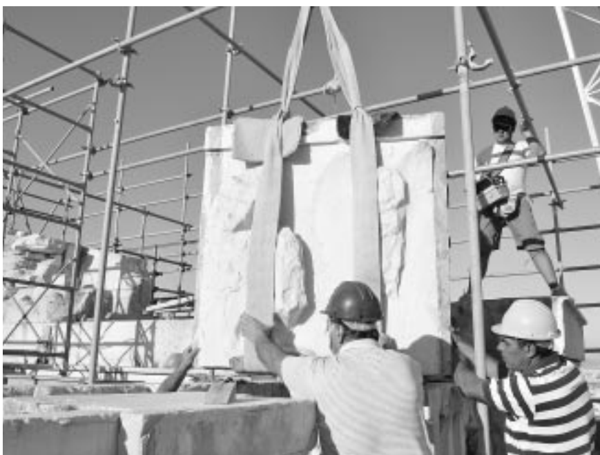
Dismantling the second from the west metope of the Parthenon north entablature. Photo V. Eleftheriou, 2011
